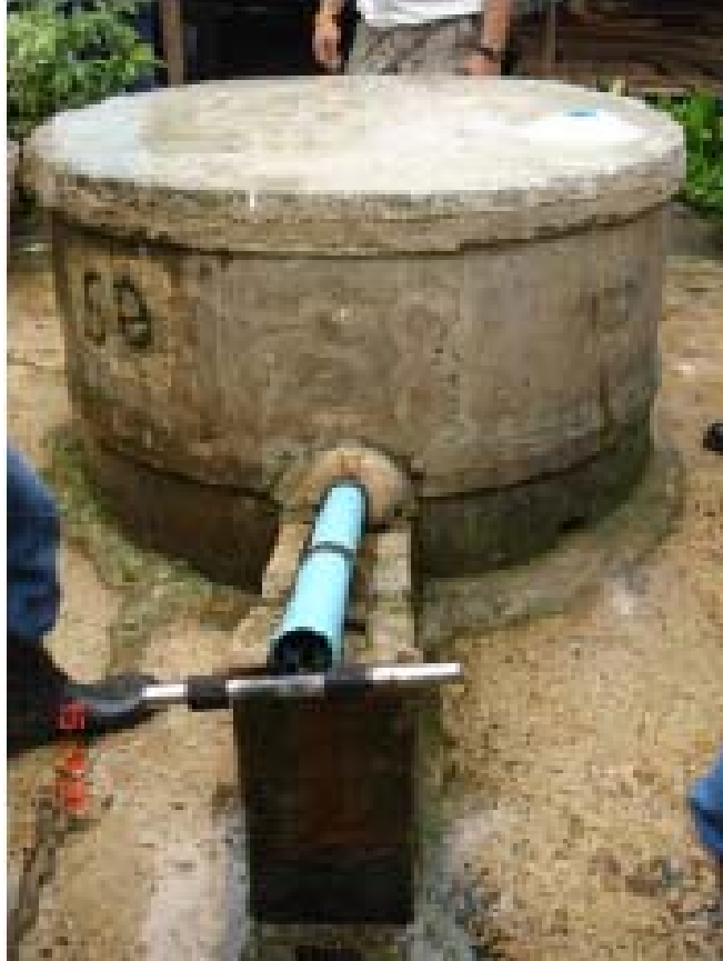
Figure 2-4: Typical rope-pump well (Lantagne, 2007).
